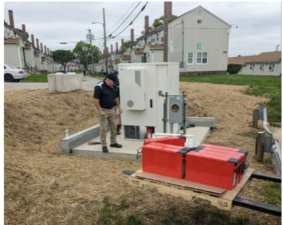
Installation of FAC unit underway at Westport Homes. (Photo Credit: BCIT, May 2024)
